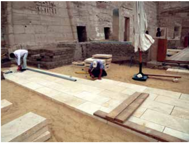
Viewing area slab laying from west. Medinet Habu. Photo by Frank Helmholz
