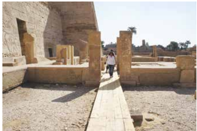
Completed wooden track for transporting materials. Medinet Habu. Photo by Ray Johnson
