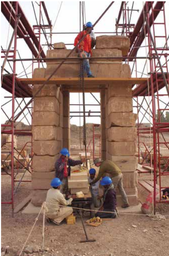
Johannes and the workmen prepare to hoist a replacement block into place on the Domitian Gate. January 8, 2016. Photo by Ray Johnson
