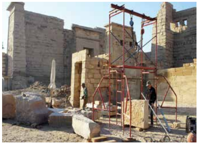
Johannes cutting stone restoration blocks outside the small Amun temple. Medinet Habu. February 3, 2016. Photo by Ray Johnson
