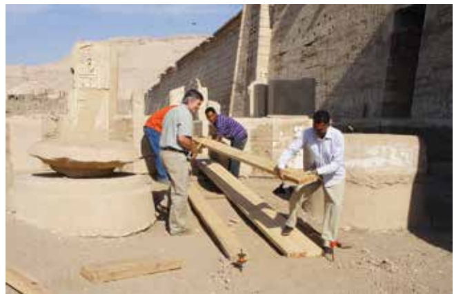
Frank and workmen creating a track for transporting materials. Medinet Habu. November 9, 2015. Photo by Ray Johnson
