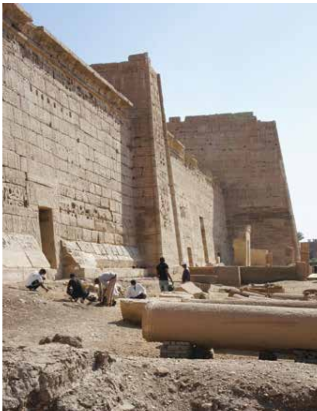
Area for restoration being cleaned. Medinet Habu. November 9, 2015. Photo by Ray Johnson
